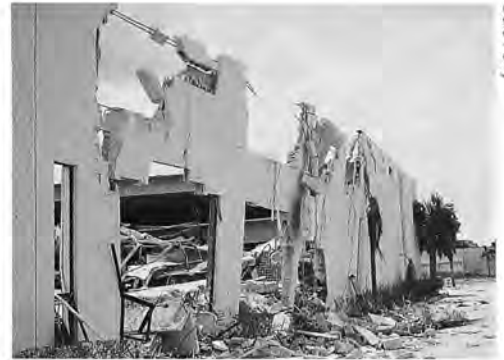
Figure 5.1: Masonry wall failure due to roof blow off.
