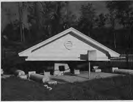
Figure 4.27: All the picnic shelters along Interstate 10 near Biloxi, MS, failed during Hurricane Elena. The shelters were in a partially protected area, but due to poor design, failed in relatively low speed winds.
