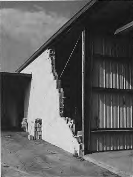
Figure 5.15: Typical infill wall failure in a pre-engineered building damaged by Hurricane Elena.
