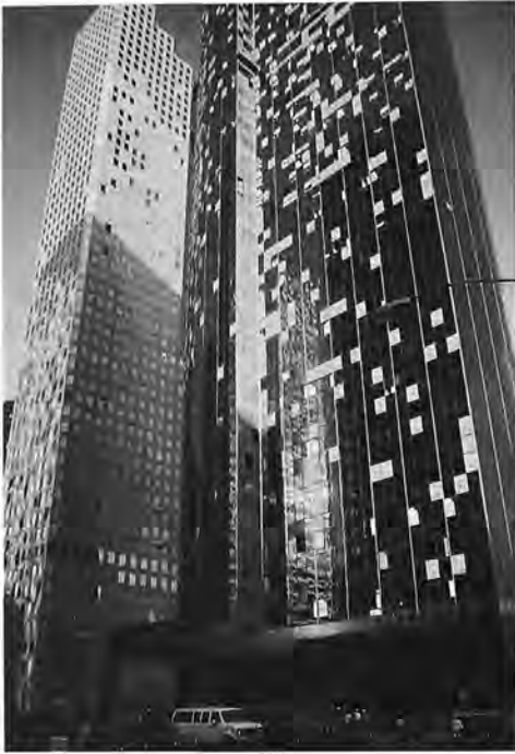
Figure 3.16: Curtain wall damage in downtown Houston during Hurricane Alicia due to wind-borne debris.
