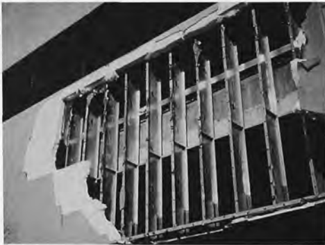
Figure 5.31: Damage to EIFS in Cutler Ridge during Hurricane Andrew.
