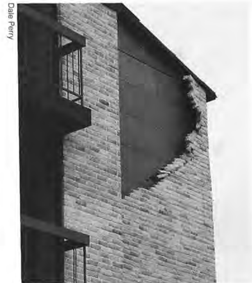
Figure 4.3: Loss of brick veneer in a tornado spawned by Hurricane Gilbert.
