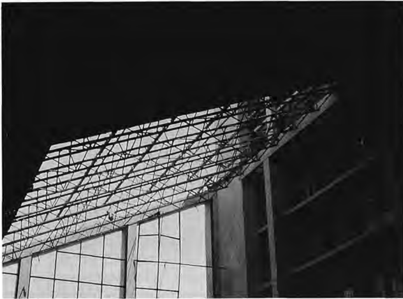
Figure 5.17: This typical pre-engineered building's roof failed in a 40 mph wind due to high internal pressure, coupled with external pressures on roof.
