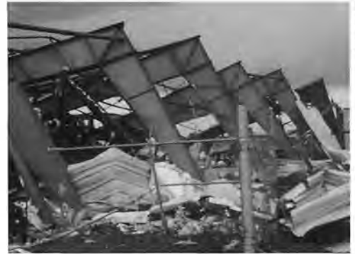
Figure 5.18: Complete collapse of metal building at Tomiami Airport, Miami, FL, from Hurricane Andrew.
