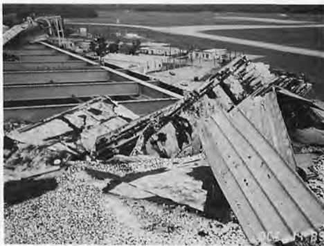
Figure 5.16: Damage to a typical pre-engineered metal roof with built-up roof.
