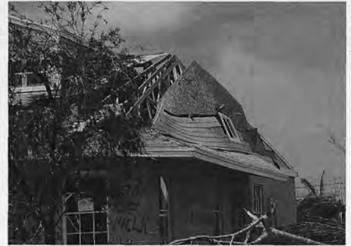
Figure 1.4: Extensive damage due to Hurricane Elena, 1985.
