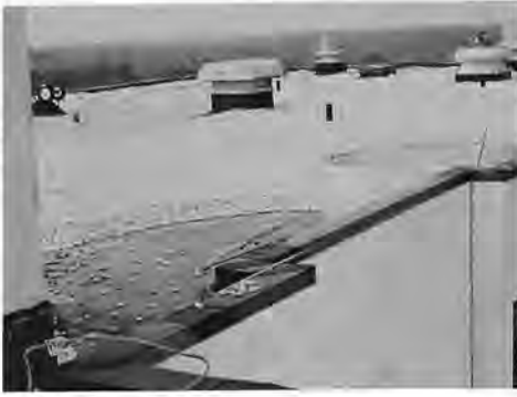
Figure 5.9: Aggregate was blown off of this single-ply ballasted membrane during Hurricane Hugo. Some fan cowlings were also blown off.
