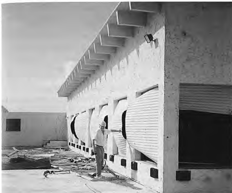
Figure 3.12: Building subjected to internal pressure as evidenced by blown-out overhead doors.
