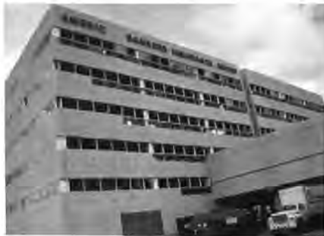
Figure 3.17: Damage in Hurricane Alicia due to wind-borne gravel ballast from roof of adjoining parking garage.
