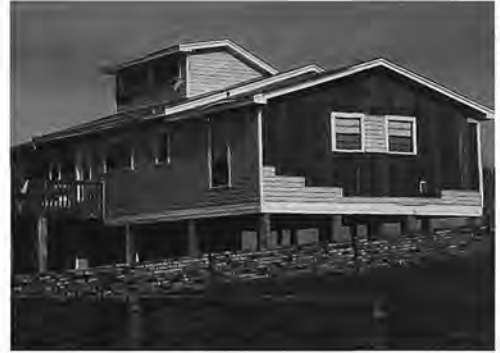
Figure 4.1: Loss of vinyl siding in wind speeds less than 70 mph, Hurricane Erin, 1995.
