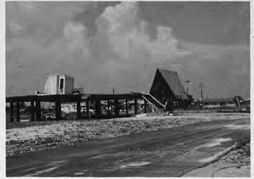
Figure 1.3: Damage on Dauphin Island, Alabama (south of Mobile) due to Hurricane Elena, 1985.
