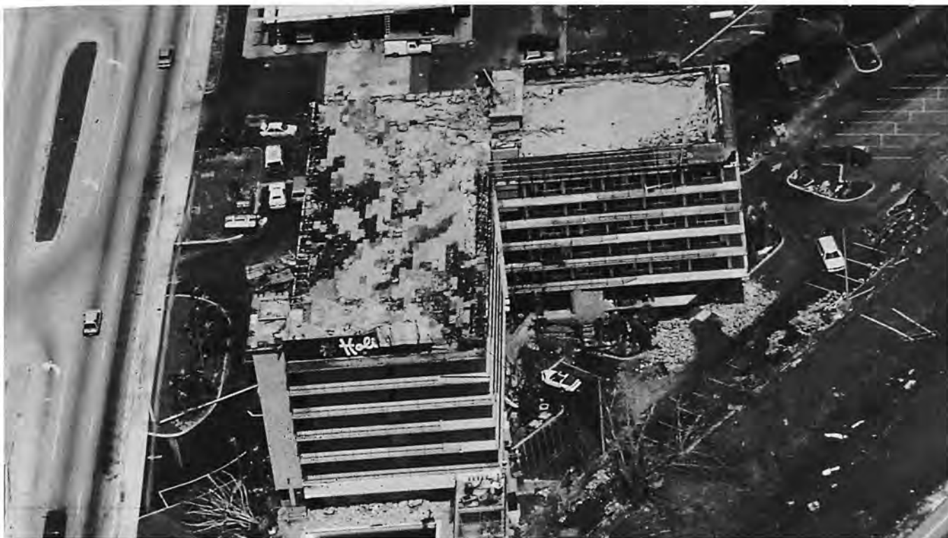
Figure 3.7: Extensive damage to roof; Cutler Ridge in Miami, FL in Hurricane Andrew.
