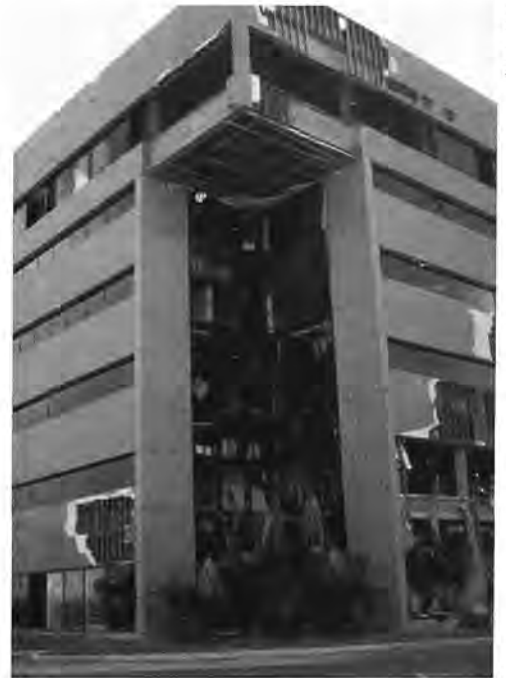
Figure 5.2: EIFS damage on a commercial building at Cutler Ridge, South Miami, FL.
