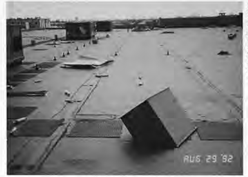
Figure 5.13: Access panels and intake hoods blew off several HVAC units during Hurricane Andrew.
