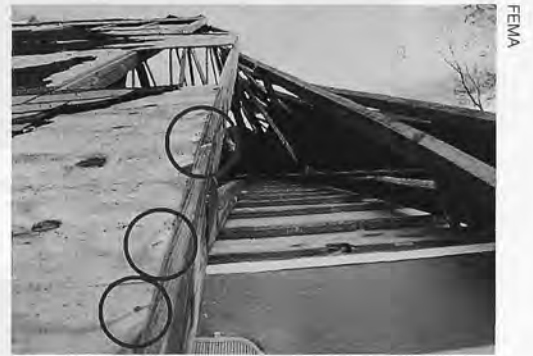
Figure 4.9: Sheathing on this roof destroyed by Hurricane Andrew was only tack nailed.
