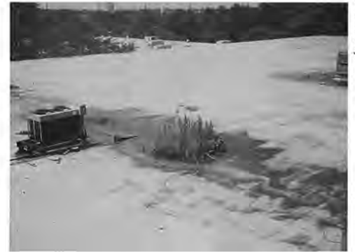
Figure 5.14: Common roof maintenance issue on a building in Long Island, NY.
