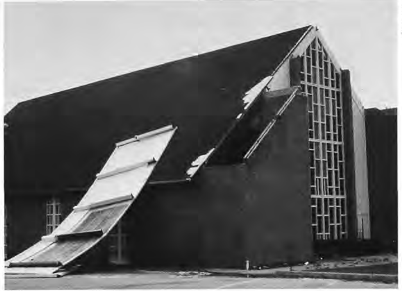
Figure 3.11: The canopy of this church in Gautier, MS suffered tremendous damage during Hurricane Elena, even though the wind speeds were only around 60 mph.
