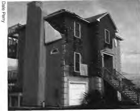
Figure 4.2: EIFS damaged in Hurricane Erin.
