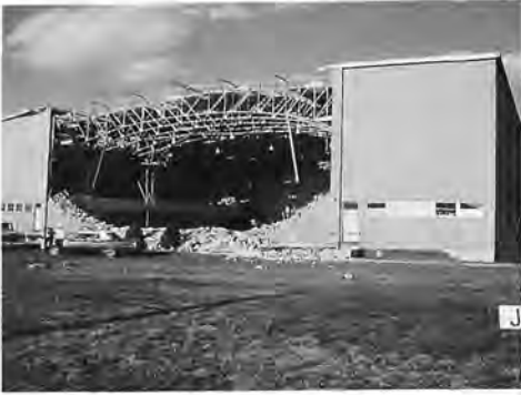
Figure 5.3: The masonry wall of this school gymnasium fell in due to positive pressure.
