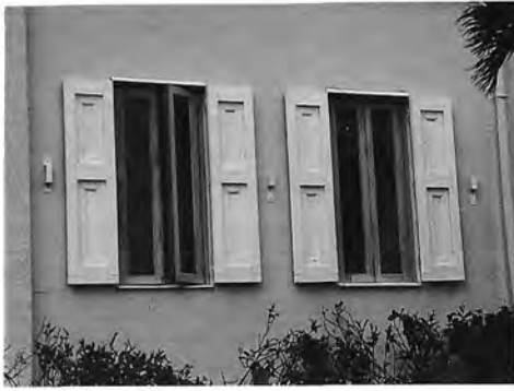
Figure 4.23: In St. Croix, Hurricane Marilyn did no damage to these shuttered windows.
